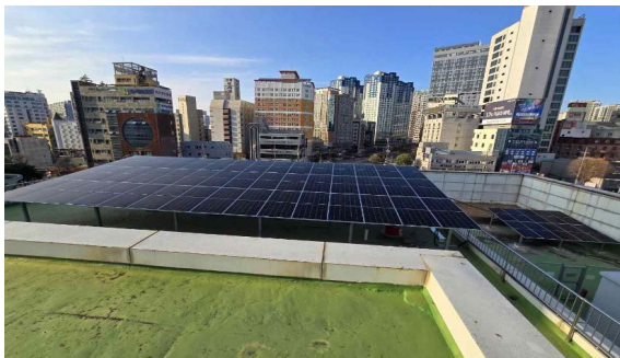
▲ Solar Panel Facilities
