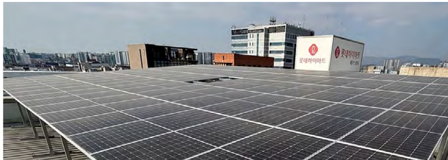
Suwon store solar panel facility
